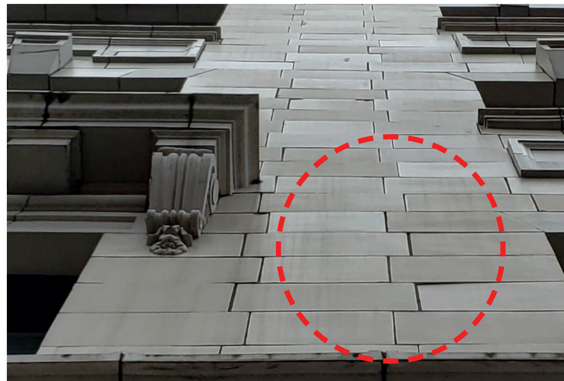
OFFSET & SPALLING TERRACOTTA
