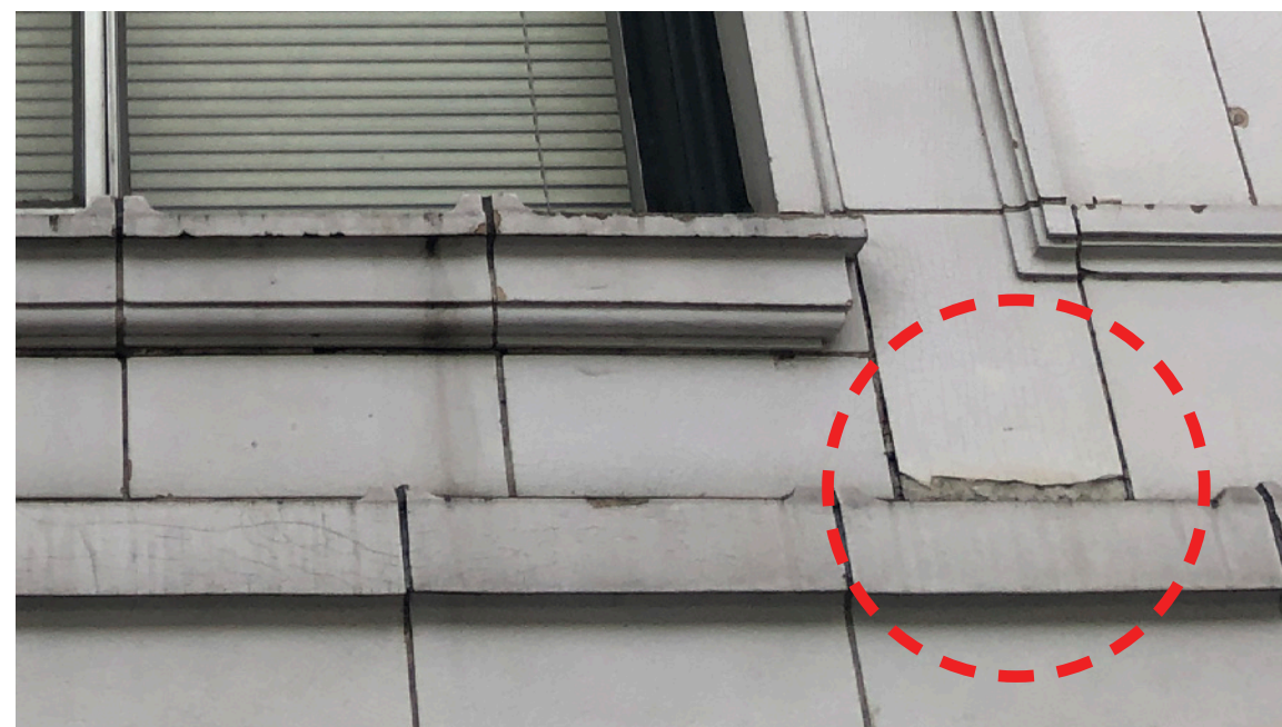
OFFSET & SPALLING TERRACOTTA
