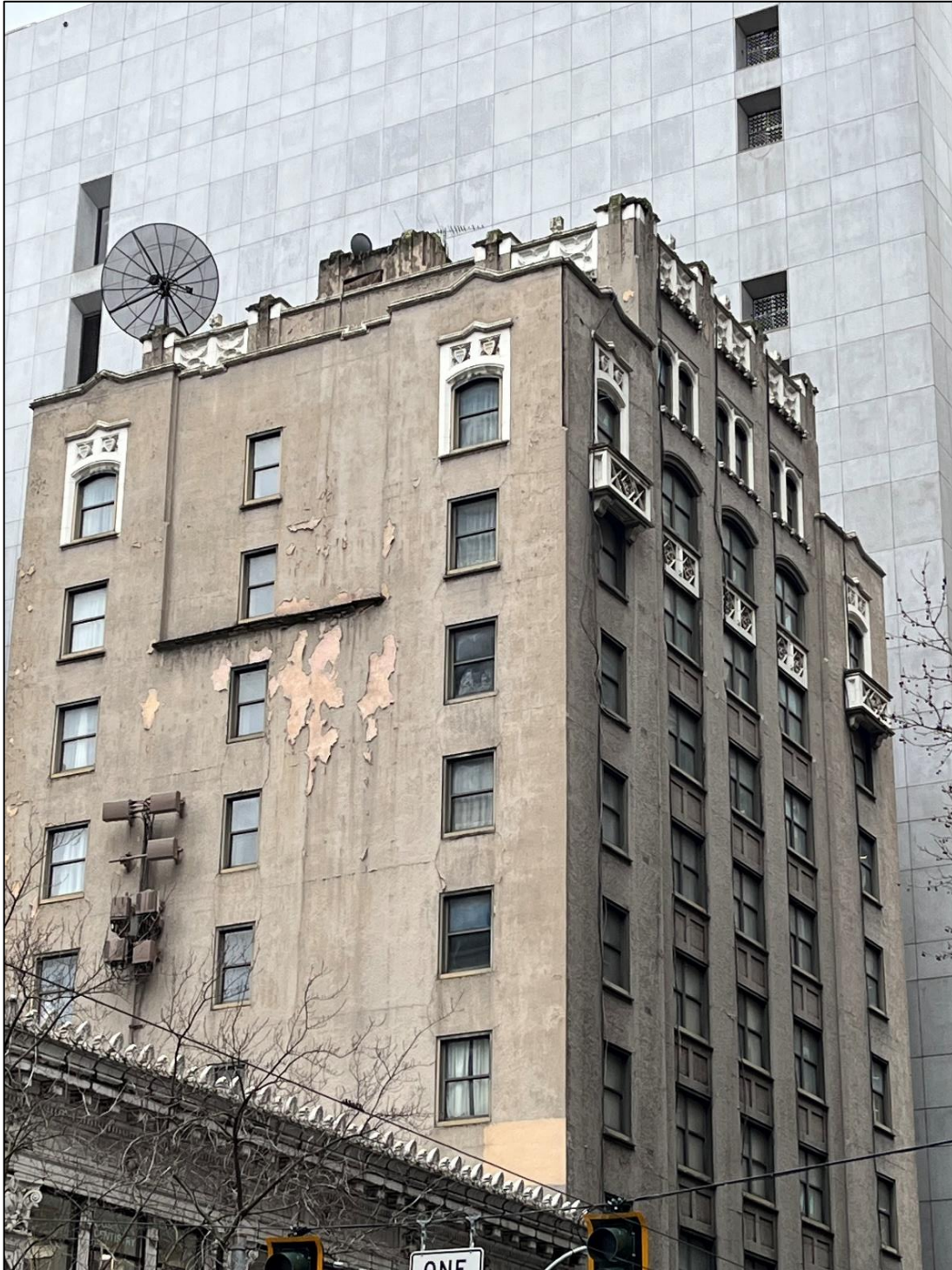
Figure 48. Looking southwest at an upper portion of the east and north facades and the uppermost setback floor.
