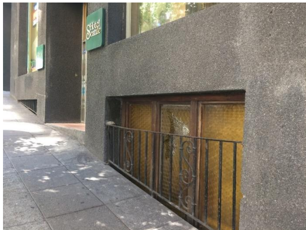
Figure 56. Below, the base and basement window along the sidewalk. Figure 57. Right, the basement entry at 315 Seneca Street. This non-original rustic style wood door, salvaged from another building, was installed in the 1960s. Canopies date from the same period.
