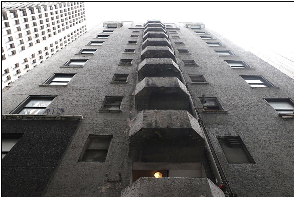
Figure 50. Below, looking upward at the west façade and egress stairs above the alley.
