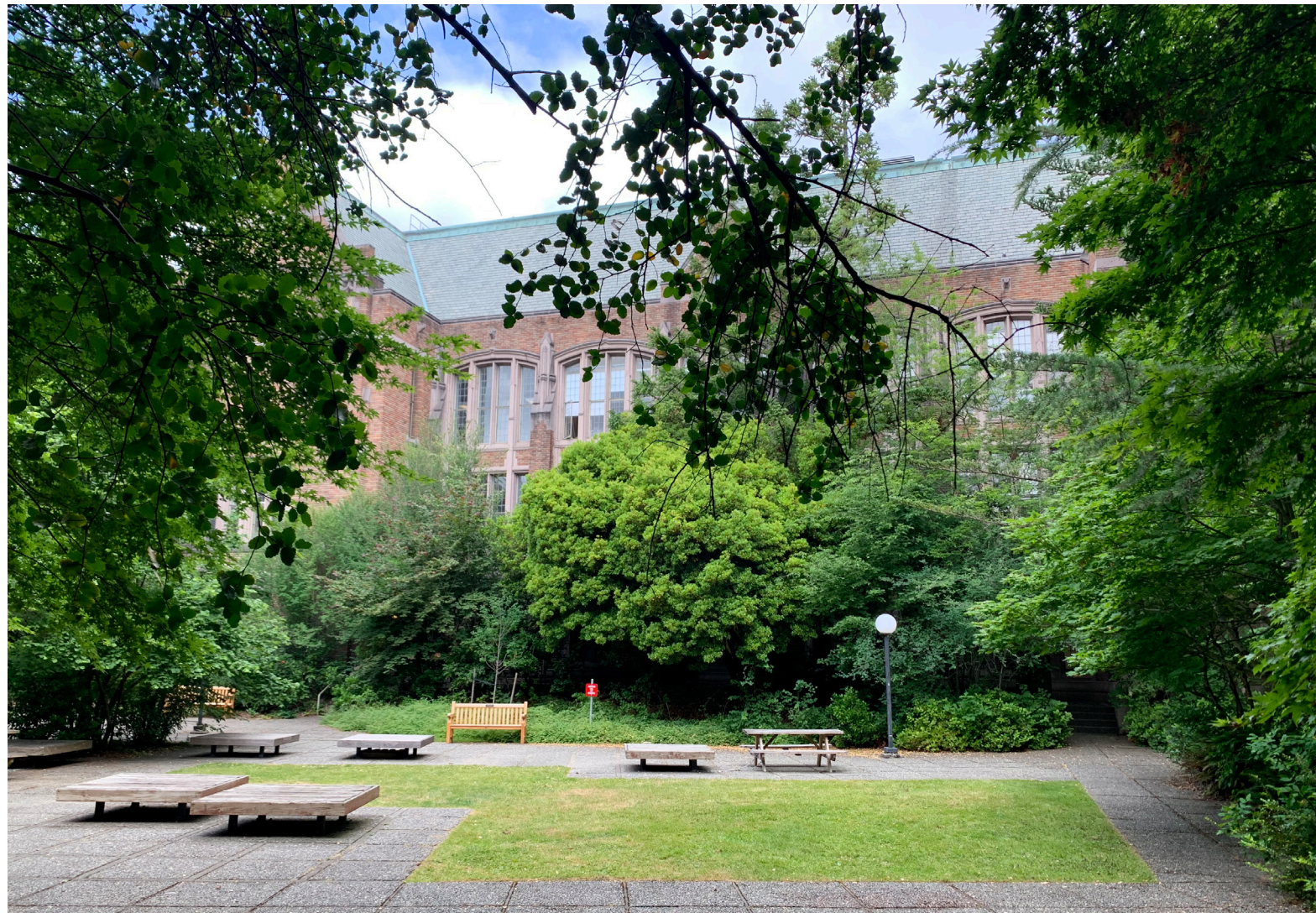
Prior to the outset of the Anderson Hall project, the south façade was substantially obscured by overgrown vegetation, diminishing the building’s presence and connectivity to the South Courtyard.
