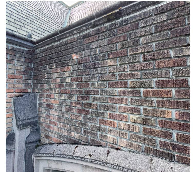
North elevation at parapet showing soiling and biogrowth on masonry, a spalled brick, and mortar deterioration at sky-facing cast stone joints.
