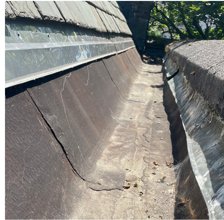
West elevation gutter showing failing liner, flashing conditions, and cast stone coping units with failing sky-facing joints.
