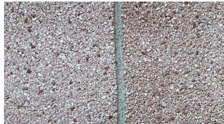
Proposed grout at new cast stone joints will match existing grout, as pictured
