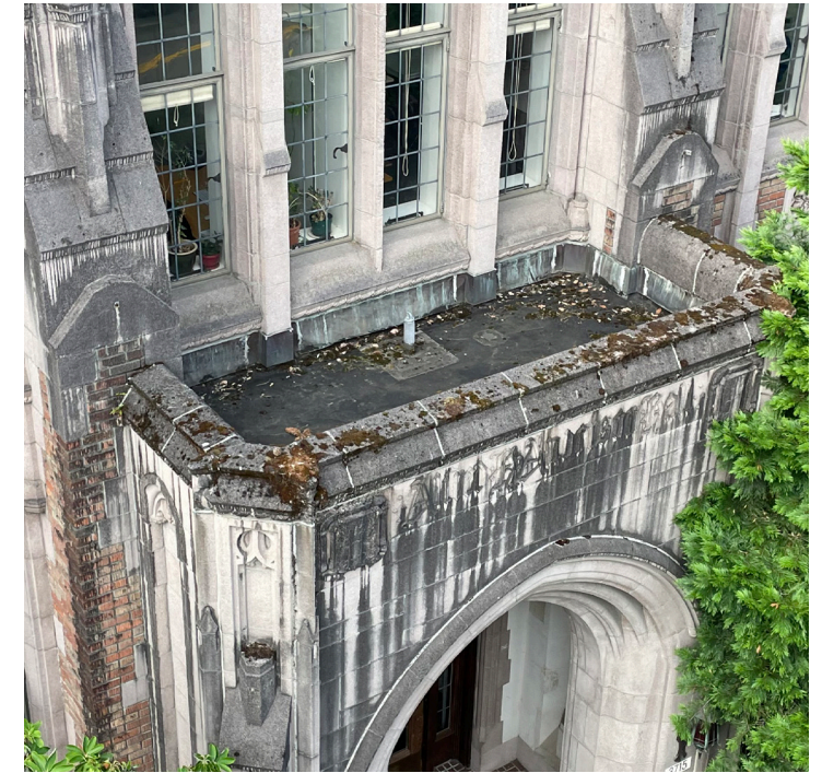
North entry parapet showing biogrowth and mortar deterioration at sky-facing cast stone joints.
