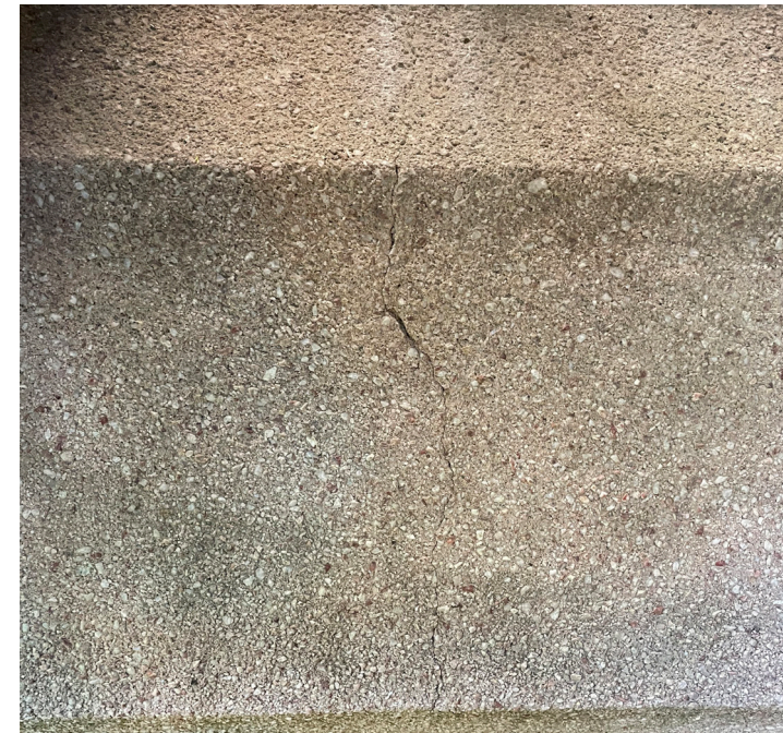
South elevation, minor crack in cast stone unit.
