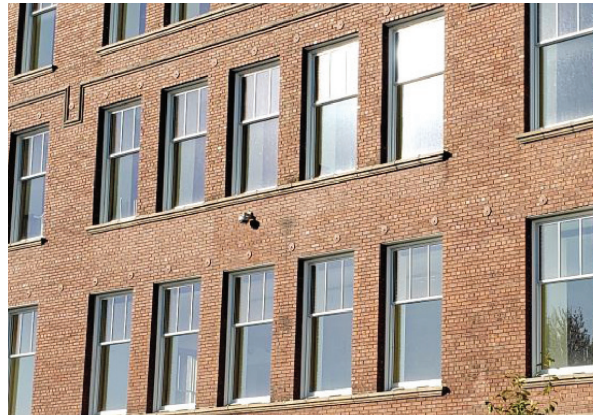
Installation of proposed security camera at Lincoln HS in Seattle
