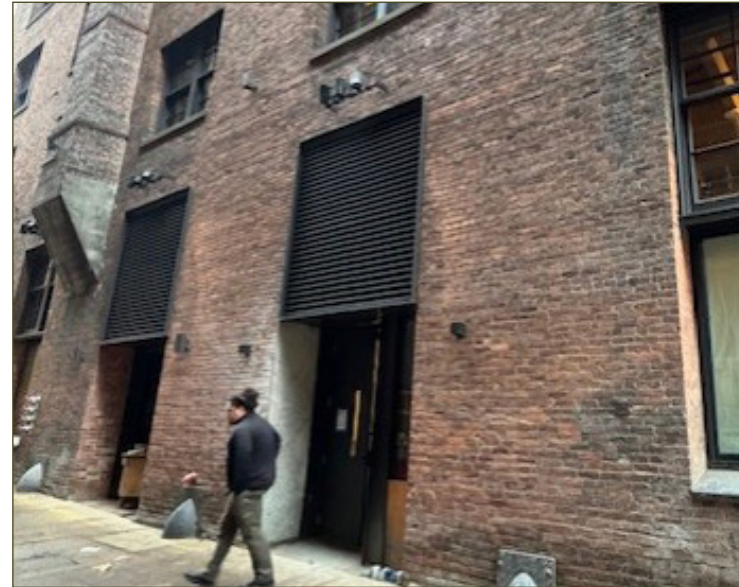
Louvers Without Adequate Clearance Behind
